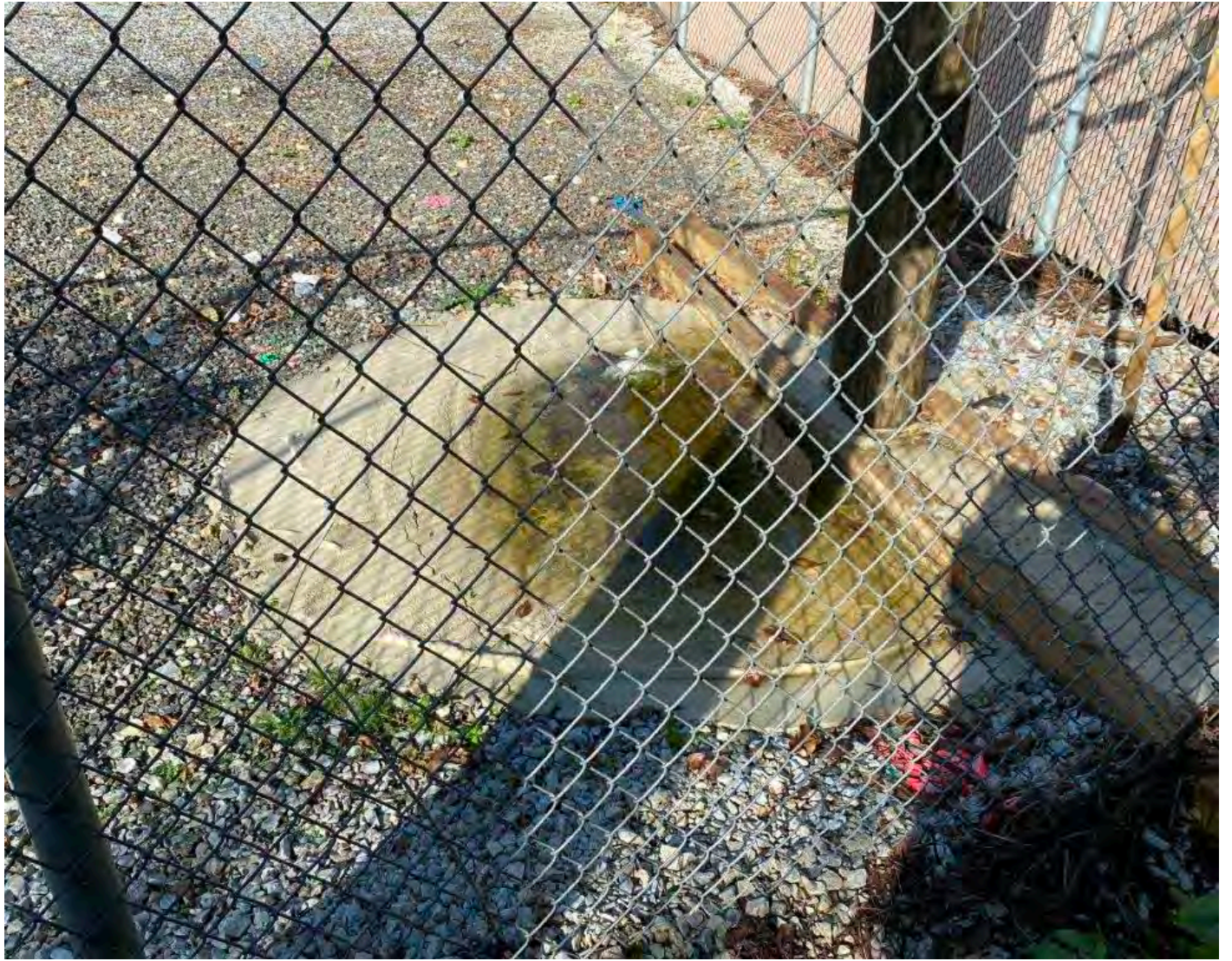
Photo 2. Recent sinkhole repaired using flowable fill inside the Sunoco valve station by the Chester Valley Trail site.
