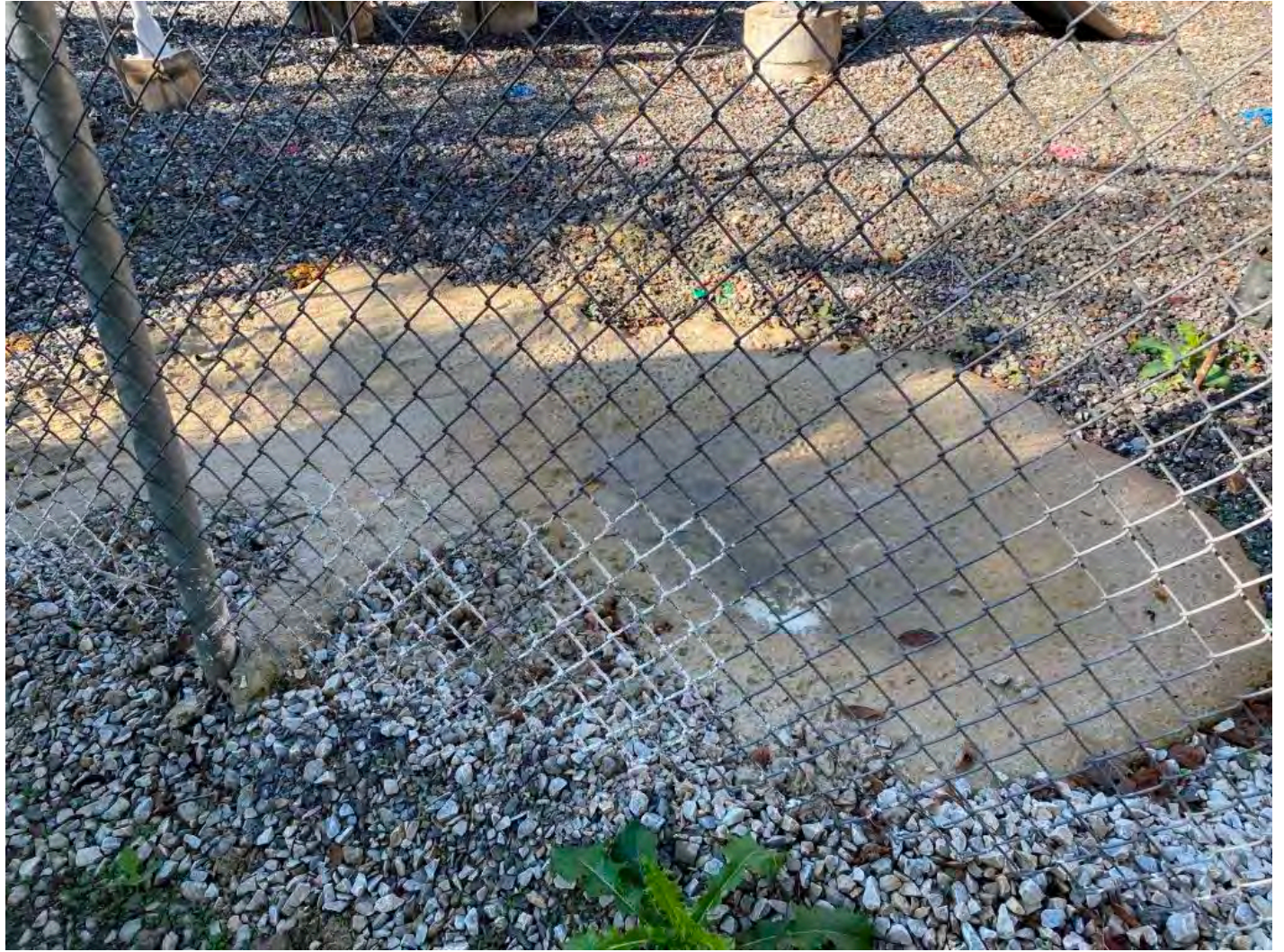
Photo 3. Second sinkhole repaired using flowable fill inside the Sunoco valve station by the Chester Valley Trail site.
