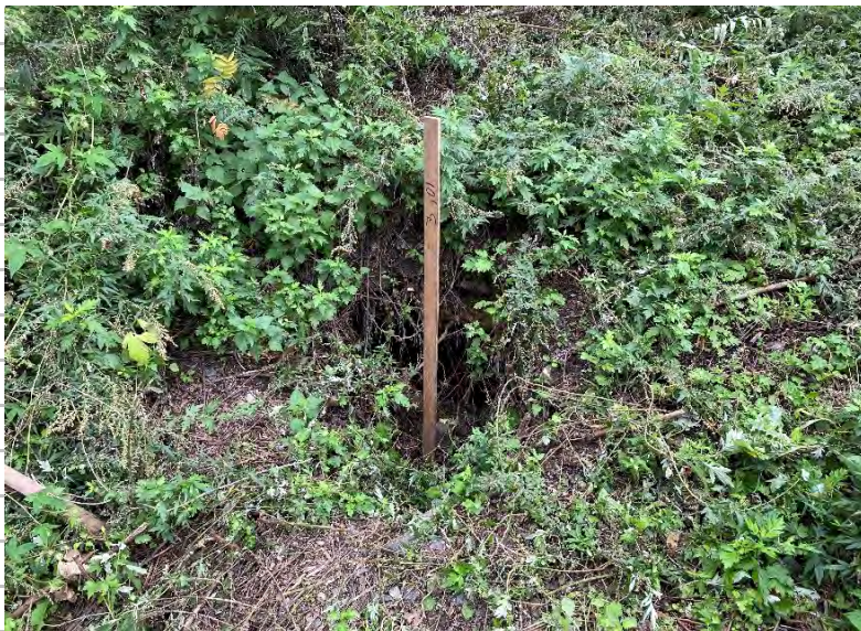
Photo 1. Recent 3' dia. x 4' deep sinkhole at toe of embankment.
