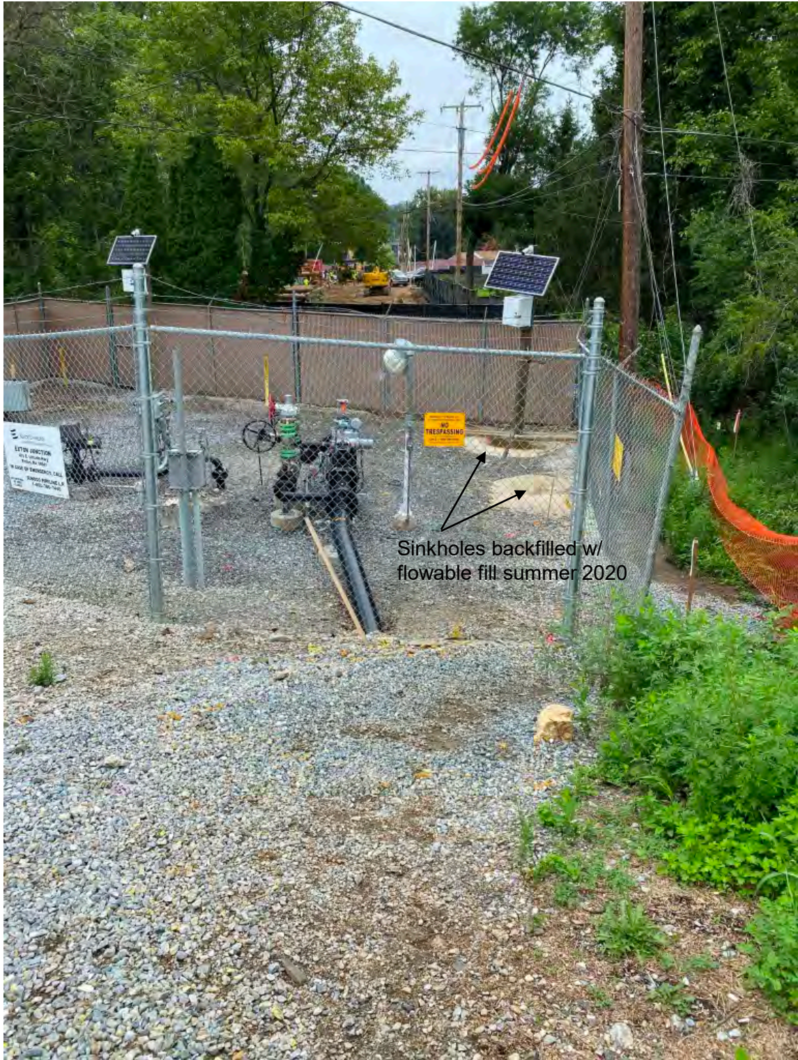
Photo 1. Sunoco valve station by the Chester Valley Trail site.
