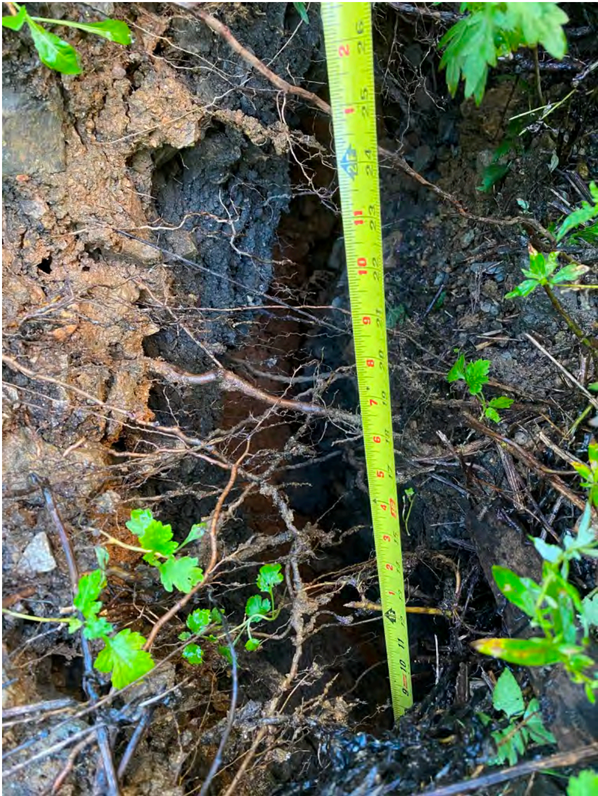
Photo 5. Close view of the new sinkhole.
