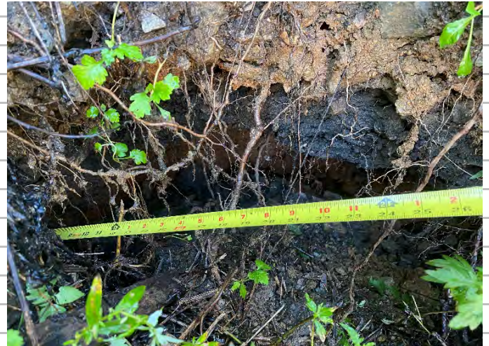
Photo 2. Close view of the recent sinkhole.
